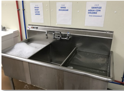
Three compartment sink setup
